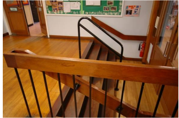
Ground floor inaccessibility to assembly hall
