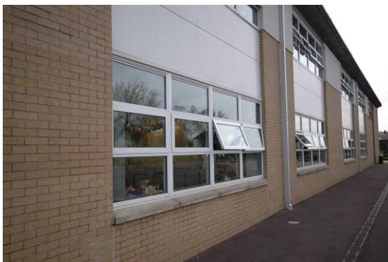
Poor opening window arrangement
