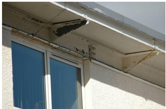
Poor detailing to roof eaves
