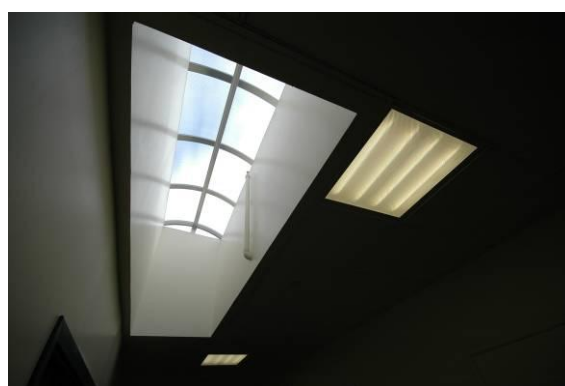
Fixed rooflights do not encourage natural ventilation
