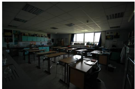
Poor glazing ratio to classroom
